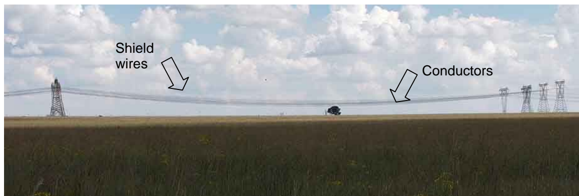
Figure 7-3: Visibility of shield wires vs. bundled conductors
