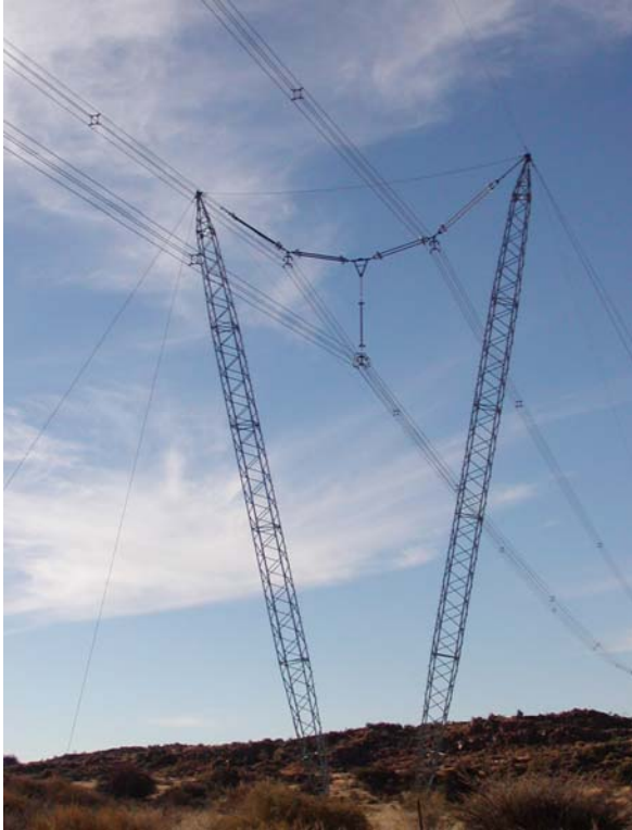
Photo 1: Cross rope suspension towers are supported by four cables attached to anchor blocks. Most of the towers will be of this type.
