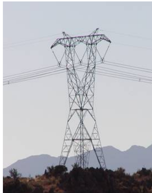
Figure 3 – Self-Supporting Suspension Tower
